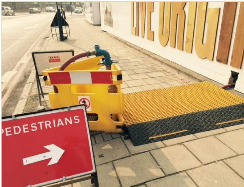
A temporary water standpipe
