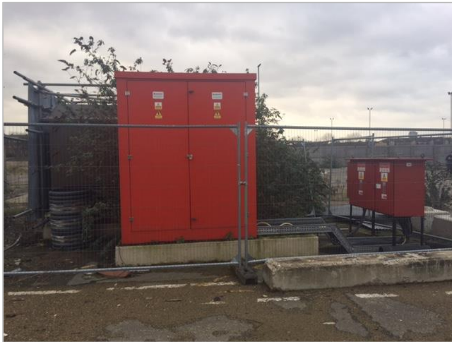
An example of a temporary electric building supply
